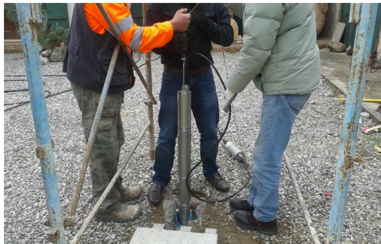
Figure 5.41 Installation of the borehole sensor at the top of the metamorphic bedrock in Site S5 (march 2014).
