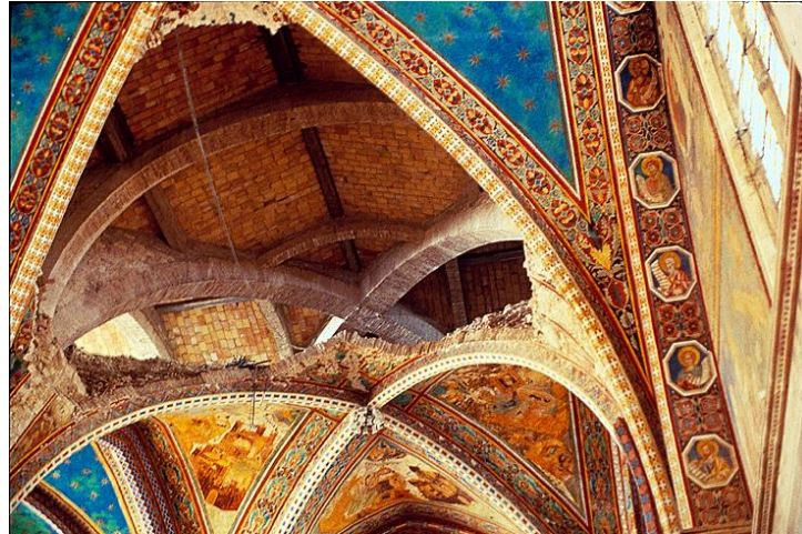
Fig. 2.5 Collapse of the frescoed vaults in Assisi, 1997
