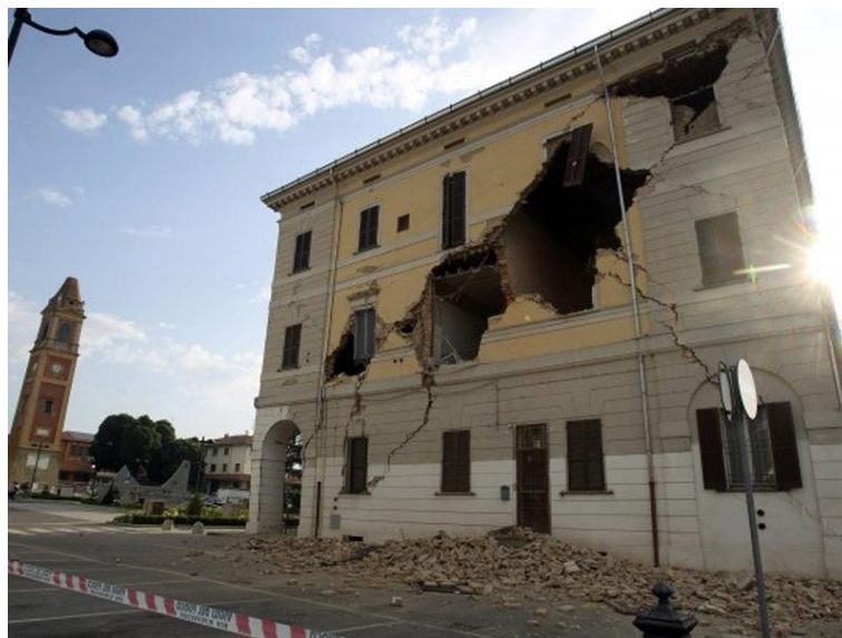
Fig. 2.8 Collapse of the facade of the Town Hall of Sant'Agostino, May 2012
