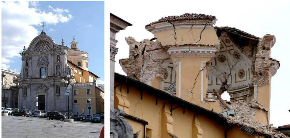
Fig. 2.7 Collapse of the Dome of the Church of Anime Sante: Before (left) and after the earthquake (right)
