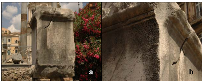
Column plinth, Trainus Market – Sampling site (a); detail of the deteriorated part (b)
