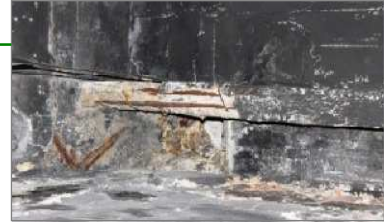
Figure 7.04 (a) Roof floor: damaged RC beam by reinforcement corrosion, in advanced state with loss of bars cross-section and concrete spalling
