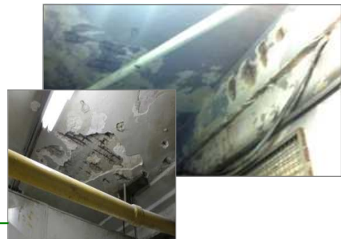
Figure 7.04 (b) Ground floor: damaged RC beam and slab by reinforcement corrosion and concrete spalling
