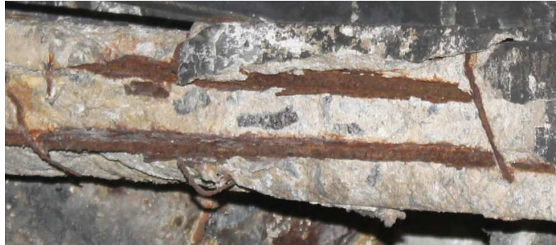
Figure 7.06 Damaged RC beam by reinforcement corrosion, in advanced state. With loss of longitudinal bars cross-section, transverse reinforcement broken and loss of concrete cross-section by spalling
