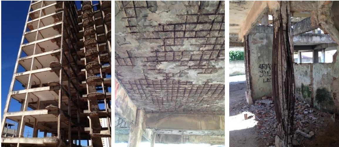
Figure 3.11 Structure in terminal state of deterioration caused by chloride attack. Extreme case of steel corrosion and concrete disintegration. Building located in the marine environment in Fortaleza city (photographs taken in May 2015)
