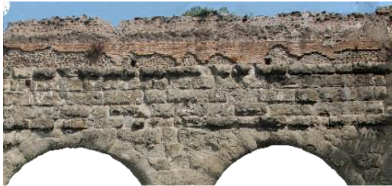
Figure 5.2 Upper channel - Anio Novus, made with ' opus testaceum ' mixed with ' opus laterazium '; low channel and arcades of Aqueduct Claudio made with ' opus quadratum '
