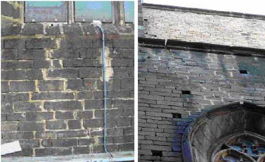
Figure 4.26 Vertical crack below windows (left) and inclined crack from windows towards tower.
