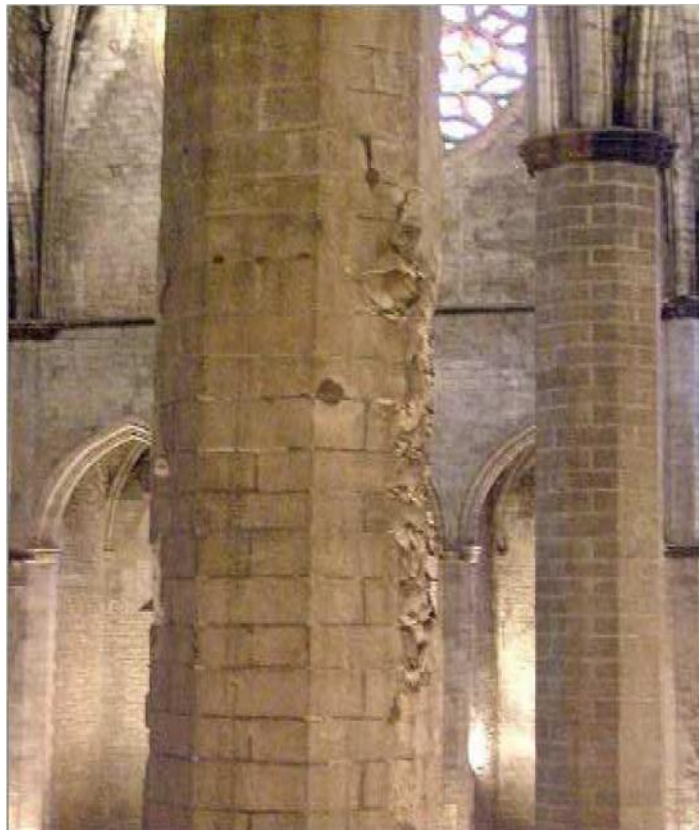
Figure 4.22 Current view of the third pier at left side, damaged due to 1936 fire.
