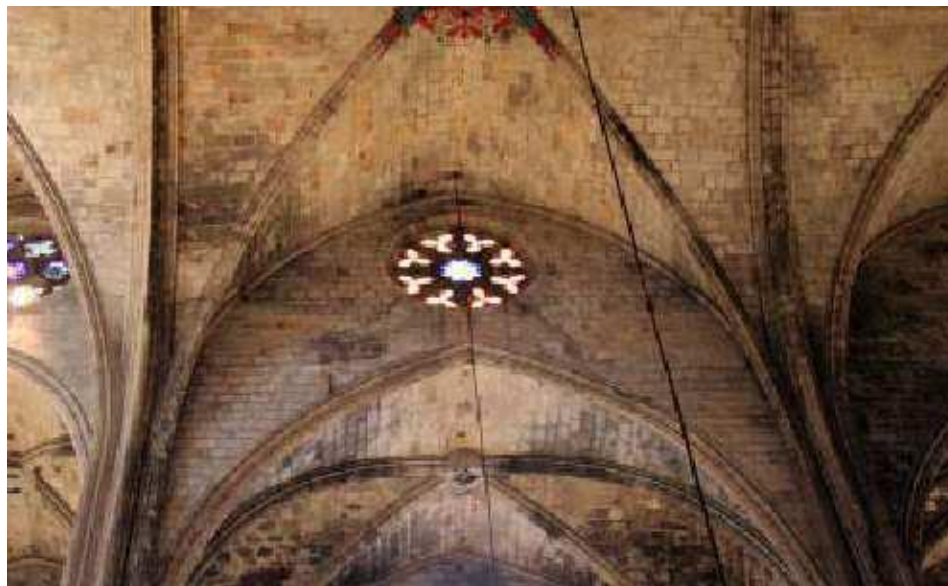
Figure 4.28 Crack in central nave.
