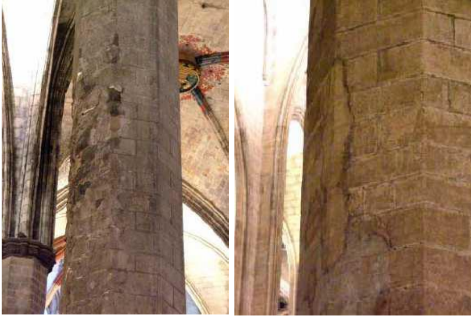
Figure 4.29 Loss of material in pier.
