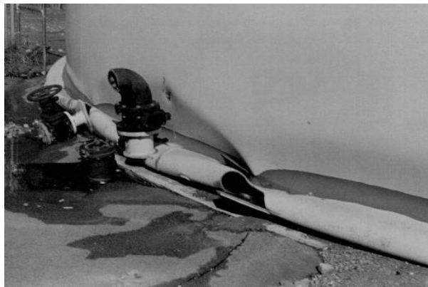
Figure 2.15. Failure of pipes attached to the tank wall (Manos Clough 1982)
