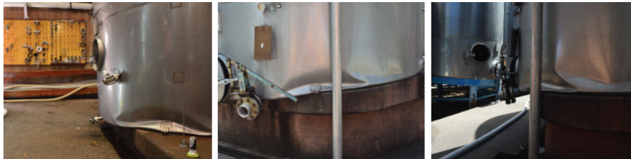
Figure 2.7. Diamond shape buckling in wine storage tanks after the 2014 Napa Valley earthquake (Fischer et al. 2016)
