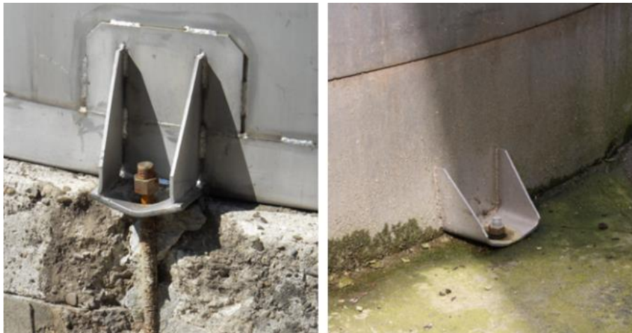
Figure 2.12. Examples of anchorage failures observed after the 2012 Emilia earthquake (Brunesi et al. 2014)
