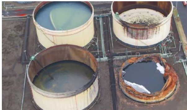
Figure 2.10. Sinking of floating roofs in two kerosene tanks at a refinery in the city of Tomakomai after the 2003 Tokachi-oki earthquake (Hatayama 2007)
