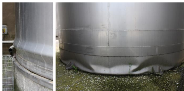
Figure 2.8. Elephant's foot buckling (left) and diamond shape buckling (right) observed after the 2012 Emilia earthquake (Brunesi et al. 2014)
