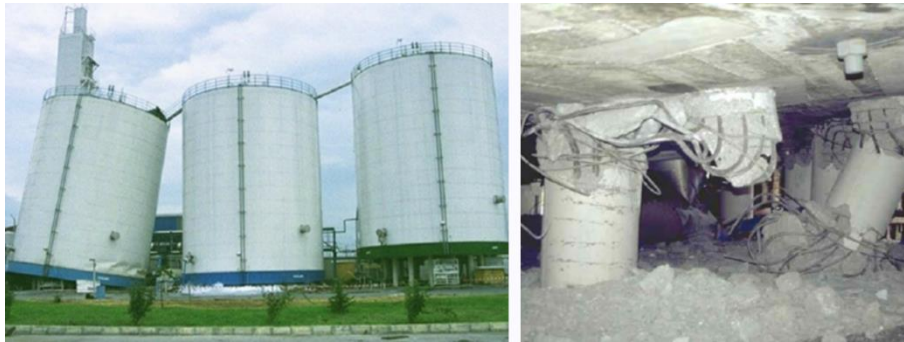
Figure 2.14. Support columns of a group of liquefied oxygen tanks collapsed after the 1999 İzmit earthquake (Sezen and Whittaker 2006)
