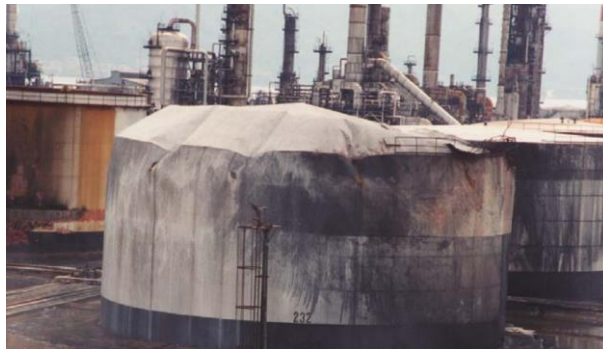
Figure 2.9. Deformation of cylindrical tank with fixed roof at the Tupras refinery after the 1999 İzmit earthquake (Sezen and Whittaker 2006)
