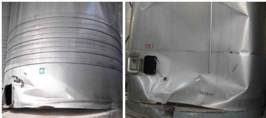
Figure 2.13. Damage caused by sliding and overturning and subsequent impact of tanks after the 2010 Maule Earthquake (González et al. 2013)
