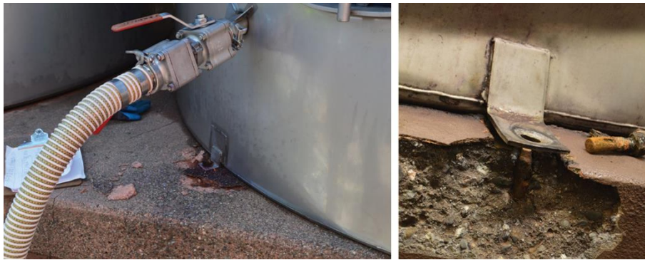
Figure 2.11. Examples of anchorage failures observed after the 2014 Napa Valley earthquake (Fischer et al. 2016)
