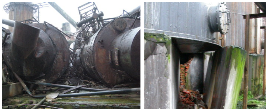
Figure 2.5. Observed damage in a chemical facility after the 2008 Wenchuan earthquake (Krausmann 2010)
