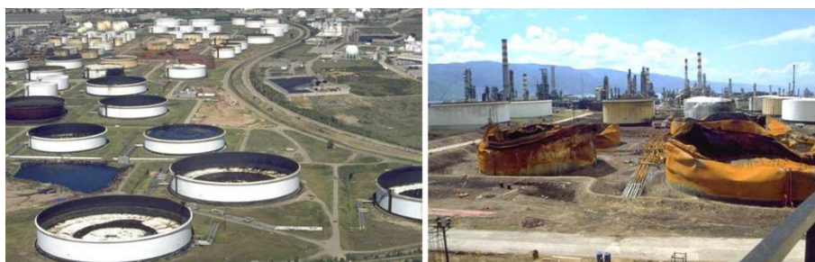
Figure 2.6. Damage to the tank farm in the Tupras refinery after the 1999 İzmit earthquake (Sezen and Whittaker 2006)
