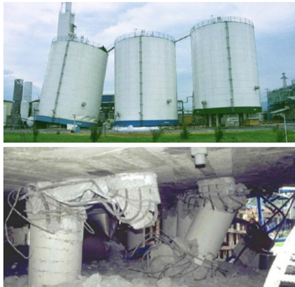
Figure 8.1. Storage tanks of liquid oxygen at the Habas plant after the 1999 Kocaeli earthquake (Sezen and Whittaker 2006)
